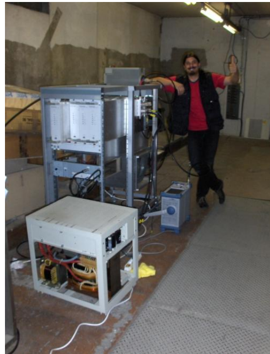
FIGURE 6 DRM transmitter and power supply
