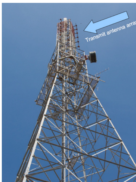
Transmitting antenna array with circular polarization
