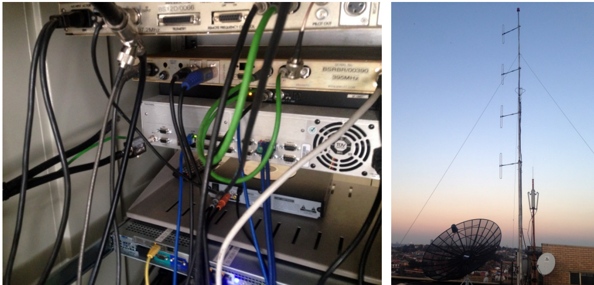
Back view of the transmitter rack and the 4-dipole antenna system with BBC C-Band reception dish:
