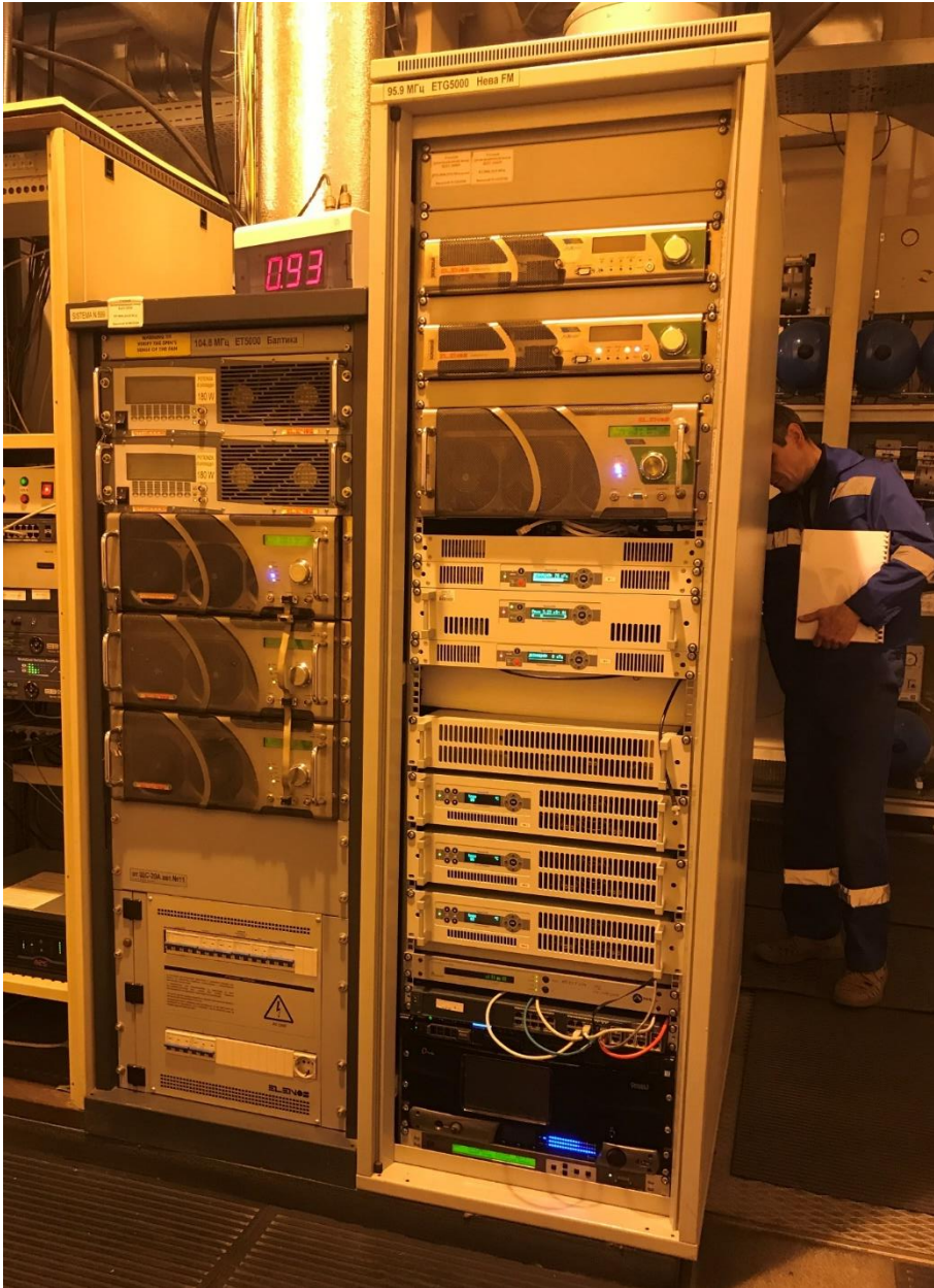
Figure 6: The DRM Simulcast transmitter, audio processor and DRM ContentServer (in the right rack cabinet below)
